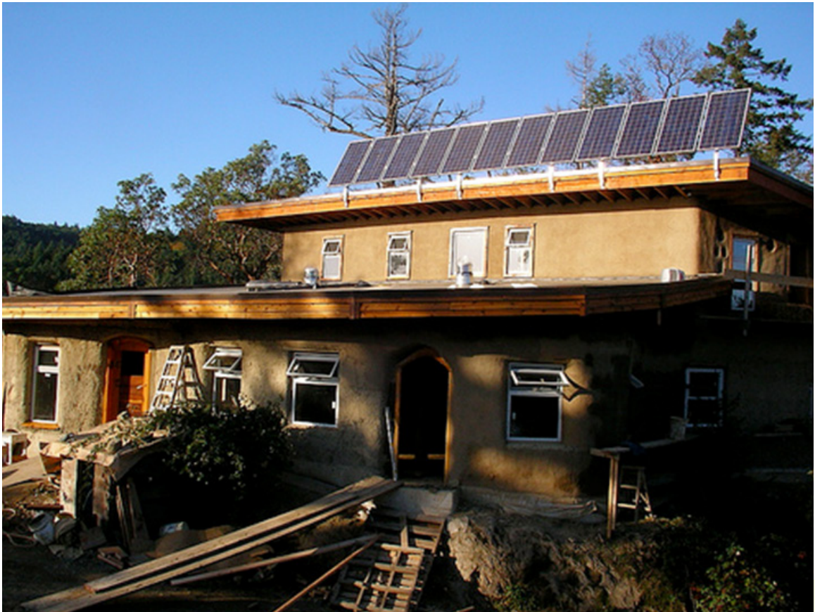
Figure 8: Eco-Sense Home (under construction) showing photovoltaic array Photo Credit Ann and Gord Baird
