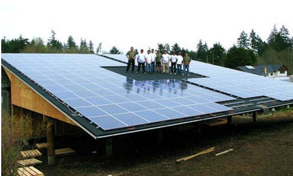
Above: A T’Sou-ke First Nation solar project.
